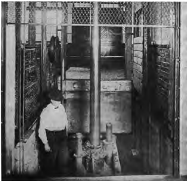
Fig. 2. Pit at Bottom of Elevator Shaft.* Note clearance to prevent person in pit being crushed; also bumpers for car and counterweight.
